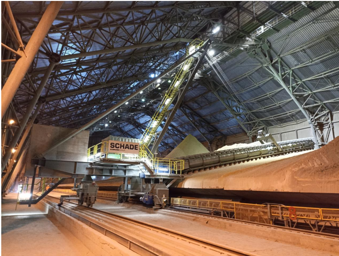
01 Precision work: SCHADE Cantilever Reclaimer with Belt Conveying equipment in operation within 10 days
