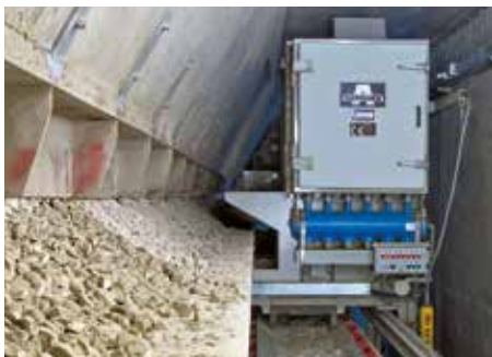
Rotary Discharge Machine (BEW)
