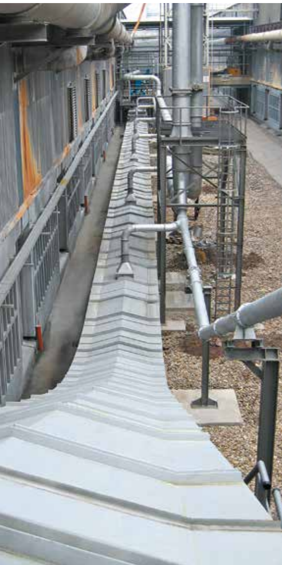
Cooling conveyor with dedusting main pipe
