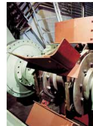
Scraper chain drive
