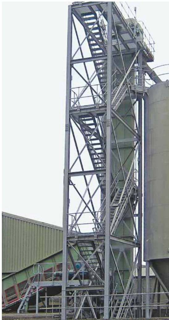
Direct transfer from Samson® to Chain Bucket Elevator
