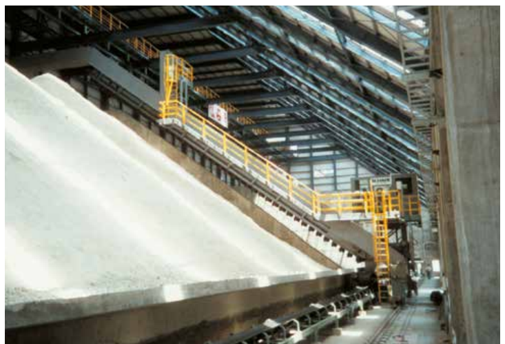
Semi-portal Scraper Reclaimer
