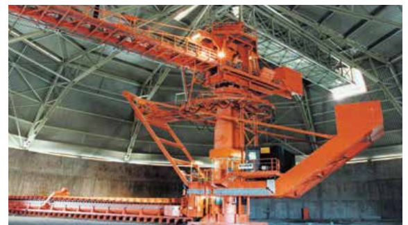
Circular Stockyard with Cantilever Reclaimer
